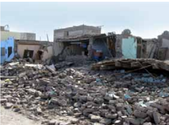
Figure 1: Dwellings that collapsed in the earthquakes in Pisco, Peru in 2007, and Maule, Chile in 2010. © J. Vargas-Neumann
