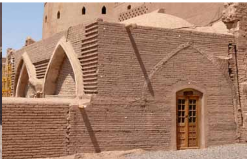
Figure 10: The stable after restoration, with arches and domes strengthened using fiberglass mesh.
