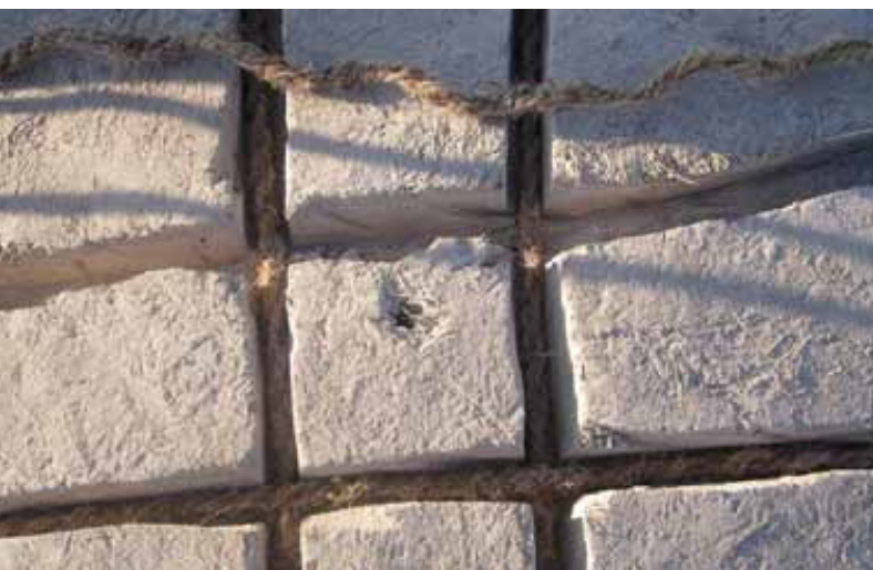
Figure 5: Detail of strengthening a dome by inserting rope made from palm fibre (SIS).
