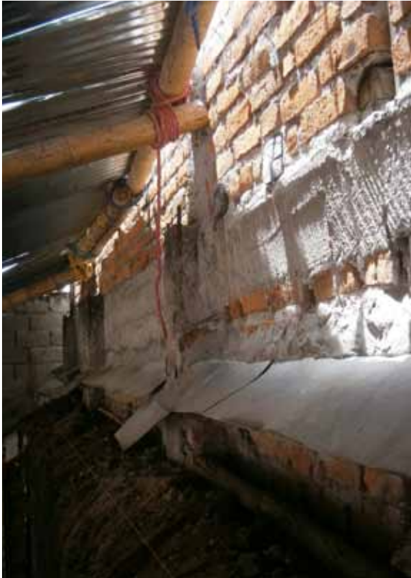
Figure 9: Common wall between the adjoining properties with concrete columns. © María de Lourdes Abad
