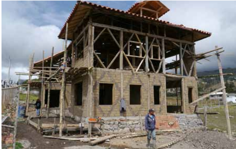
Figure 11: Second wattle and daub house in Cañar, with a structure of recycled eucalyptus poles, bamboo canes and mud filled with compressed earth blocks. © María de Lourdes Abad
