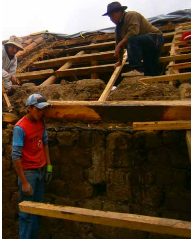
Figure 10: Tile roof with wood, bamboo and mud support structure. © María de Lourdes Abad
