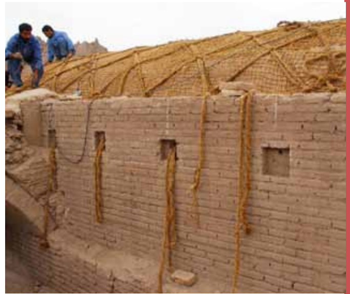
Figure 8: Strengthening an arched roof with rope and mesh made from palm fibre (SIS).
