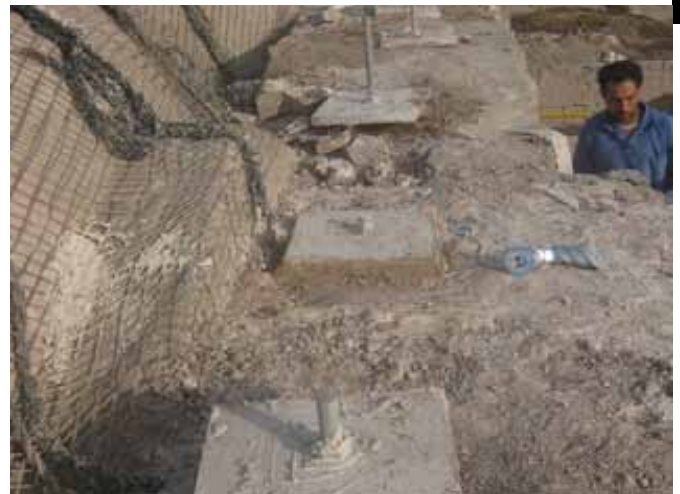
Figure 2: Strengthening the join between a pillar and an arch with Geogrid mesh and plastic (Teflon) plate.
