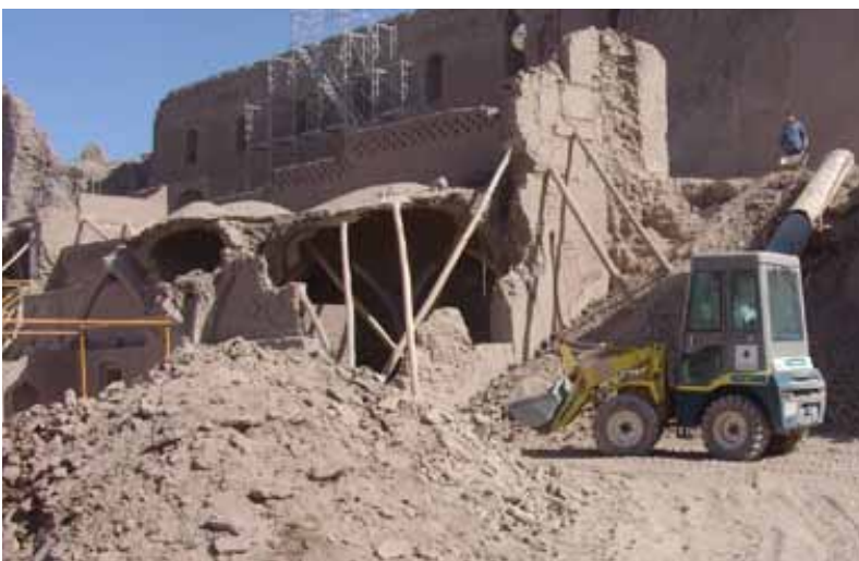
Figure 9: The stable immediately after the earthquake.
