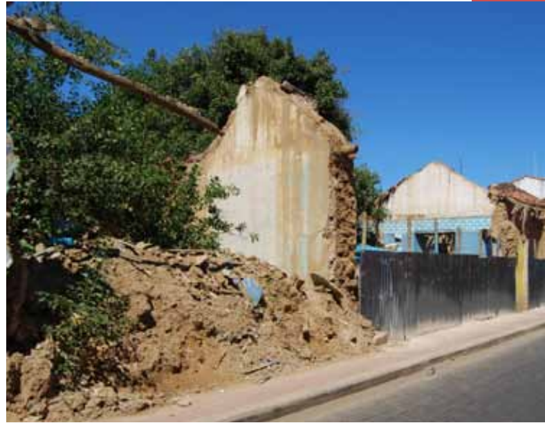
Figure 7: Collapse of an uninhabited house, Coro. © L. Guerrero
