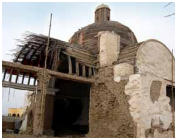
Figure 5: Avoid reinforcements based on beams and reinforced concrete columns, as their different behaviour in earthquake conditions can lead to collapse rather than protect the adobe walls. Damage to the San Luis de Cañete Church in the Pisco earthquake of 2007. © J. Vargas-Neumann
