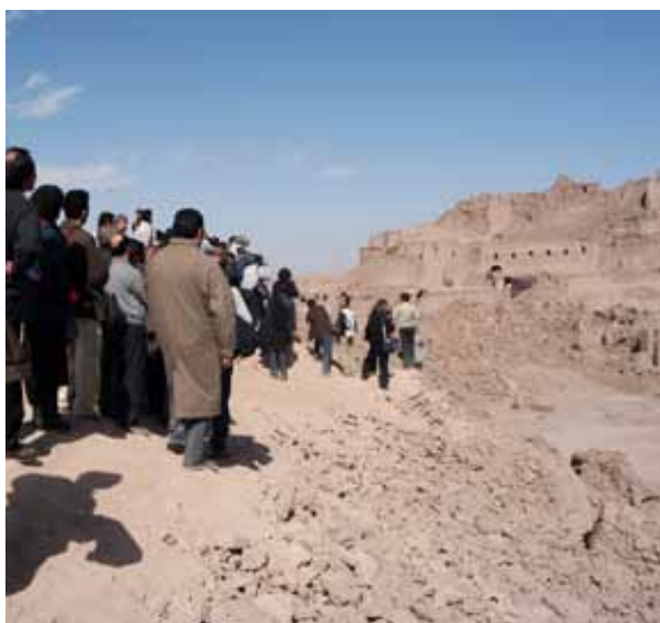
Figure 6: The quantity of visitors posed a challenge in the first days after the earthquake. © Afshin Ebrahimi/Seyed Hadi Ahmadi Roini
